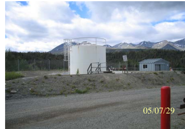
Photo 0135: 3440 Bulk fuel storage tank with geomembrane and berm
