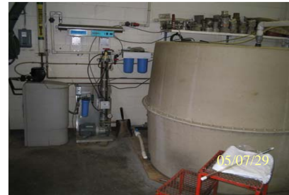
Photo 0132: 3440 Water storage tank (right), duplex filter (centre), UV disinfection system (top centre), reverse osmosis treatment system (bottom centre), water softener (left)
