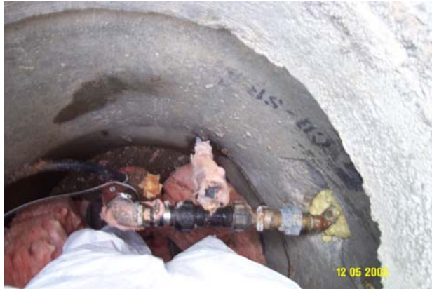
Photo 0144: M0093 Wellhead in Pit
