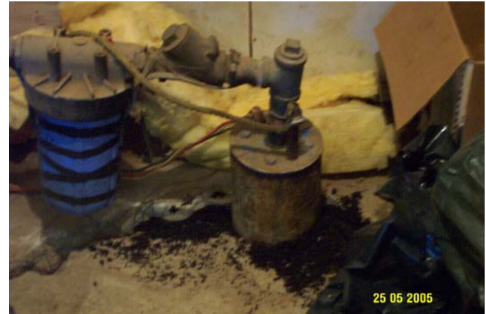
Photo 0197: 6512 Wellhead (center) and Filter (left)
