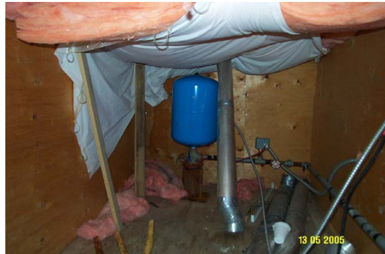
Photo 0167: M0201 Wellhead and Pressure Tank
