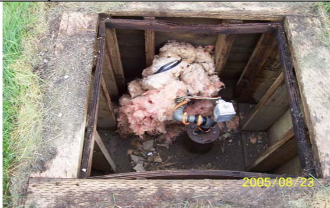
Photo 379: M0156/M0226 Well enclosure and wellhead.
