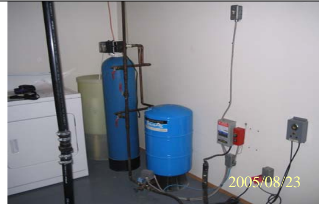
Photo 199: M0156/M0226 Water System (pressure tank, pump controls, softener).
