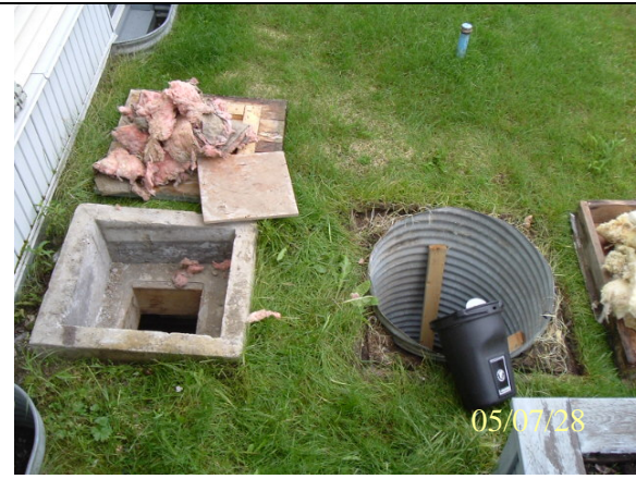
Photo 0570: 3100 Wellhead in pit (right), access enclosure (left)
