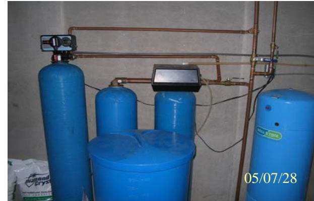
Photo 0103: 3100 Wellhead in pit (right), access enclosure (left)
