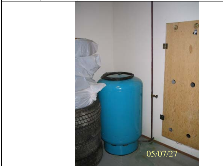
Photo 0089: M0133 Pressure tank
