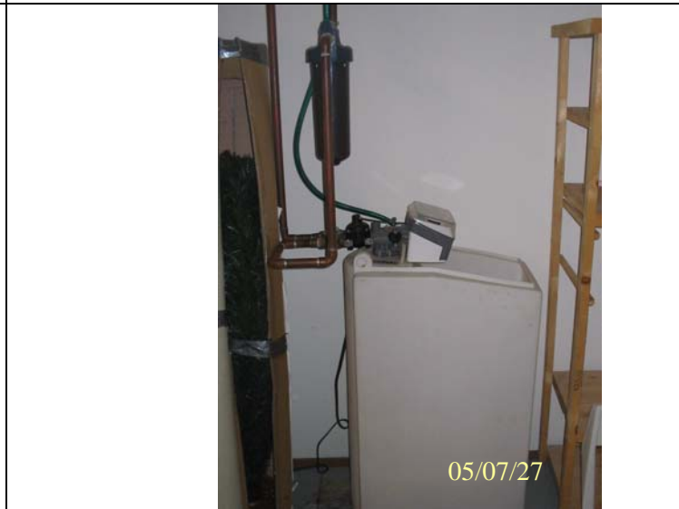
Photo 0090: M0133 In-line filter and water softener
