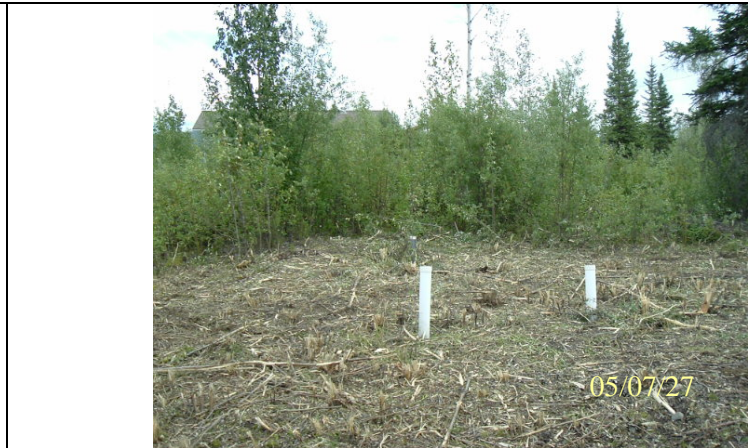
Photo 0544: M0133 Septic field
