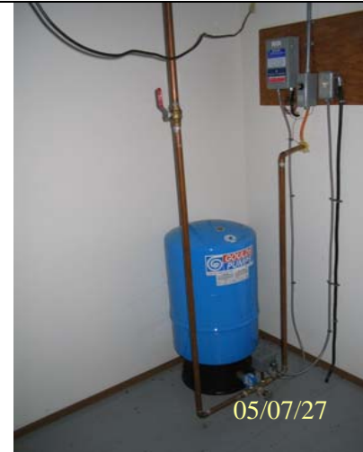
Photo 0094: M0134 pressure tank and pump controls
