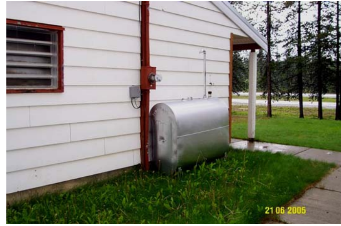
Photo 0282: M0092 Above ground fuel storage tank
