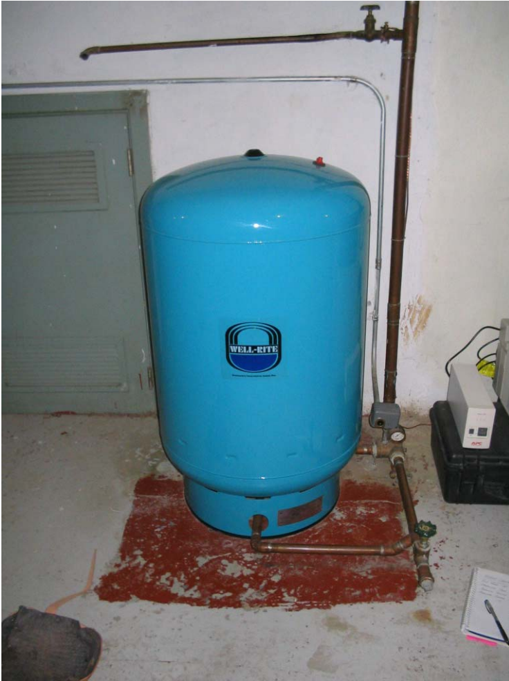
Photo 0022: M0092 Pressure tank
