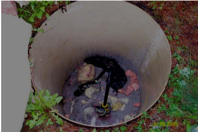
Photo 0281: M0092-A Wellhead in pit
