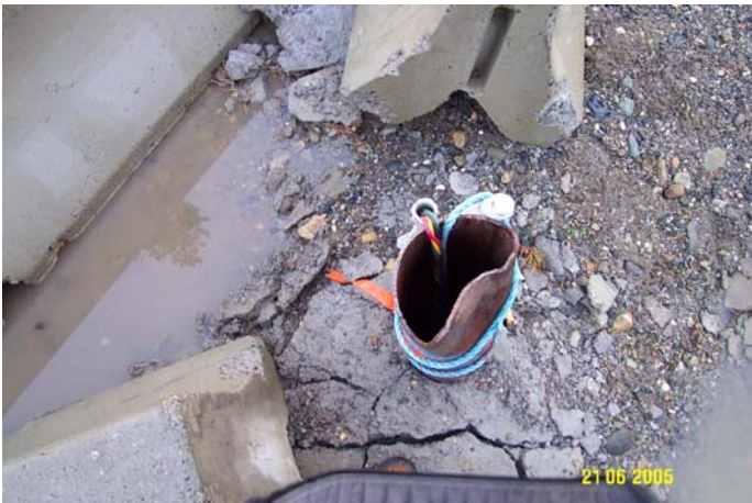
Photo 0288: 4821 Wellhead – notice damage due to impact with truck
