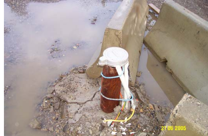
Photo 0290: 4821 Wellhead – pitless adapter
