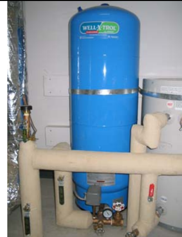
Photo 0023: 4821 Pressure tank and controls
