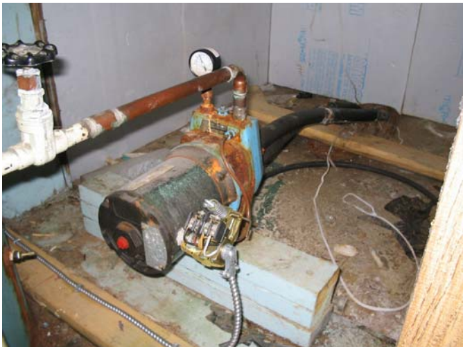
Photo 0043: M0086 Wellhead (back right), and jet pump (front centre)
