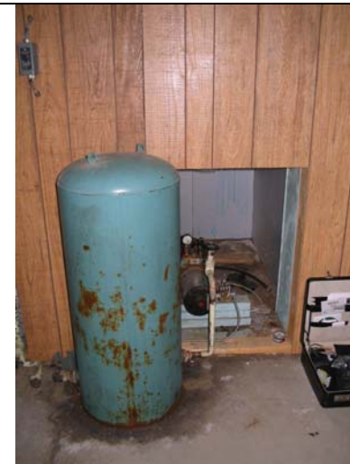
Photo 0044: M0086 Pressure tank (left) and wellhead enclosure off of basement of residence
