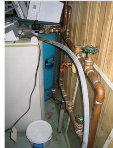
Photo 0034: M0088 Water softener (left), and pressure tank (behind)
