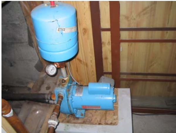
Photo 0032: M0088 Jet pump and pressure tank
