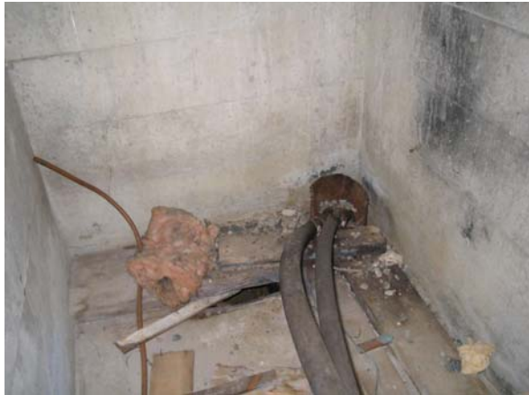
Photo 0033: M0088 Wellhead in concrete enclosure off from basement of residence
