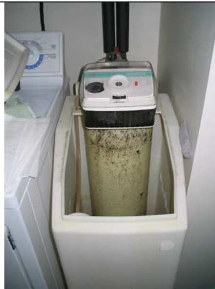
Photo 0039: M0127 Water softener
