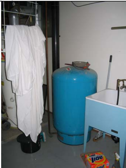
Photo 0038: M0127 Pressure tank
