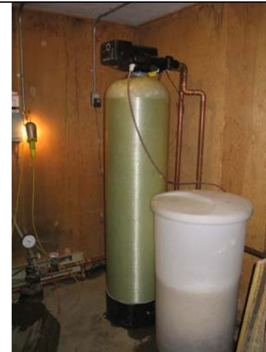
Photo 0018: 4836 Water softener and brine tank
