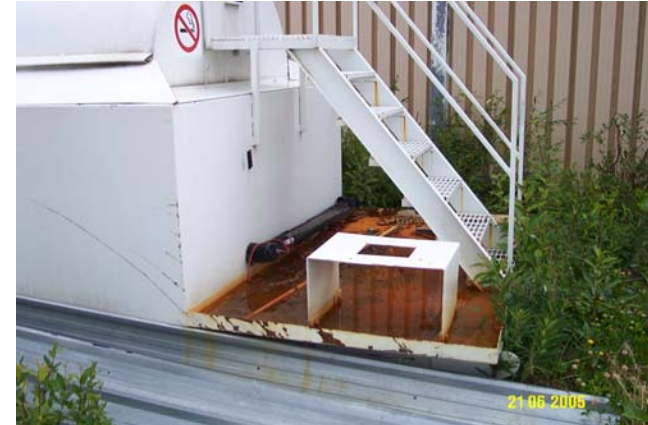
Photo 0275: 4836 Above ground fuel storage tank
