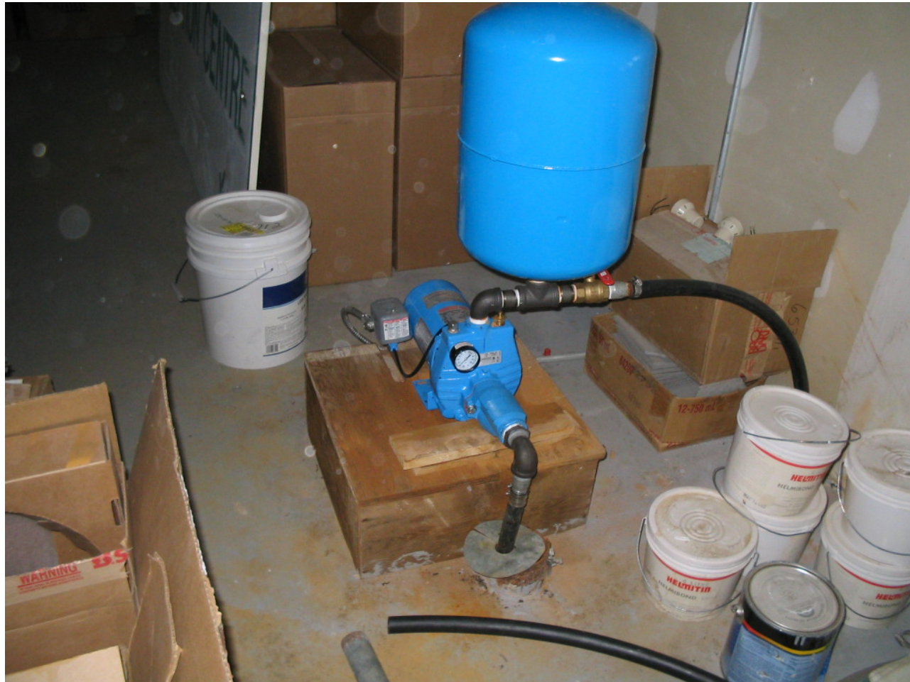
Photo 0030: 4841 Well (centre), jet pump (behind well), and pressure tank (behind jet pump) in basement of Visitor Reception Centre – system not currently in use
