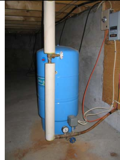
Photo 0237: 4842 Pressure tank (centre) and pump controls (right)
