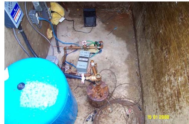
Photo 0260: 4840 Wellhead (centre), and pressure tank (left) in enclosure
