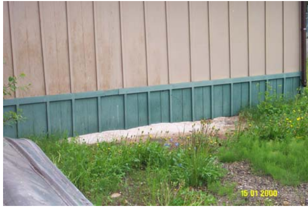
Photo 0264: 4840 Absorb-all on ground behind office building – likely site of hydrocarbon contamination
