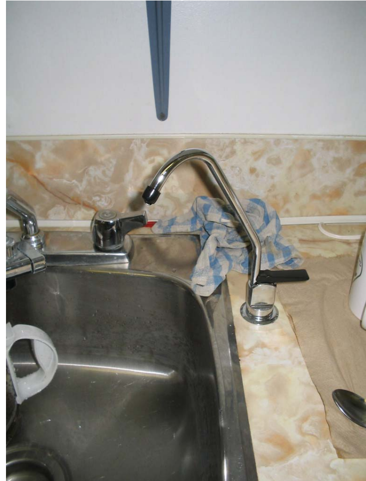
Photo 0007: 4840 Reverse osmosis tap in kitchen
