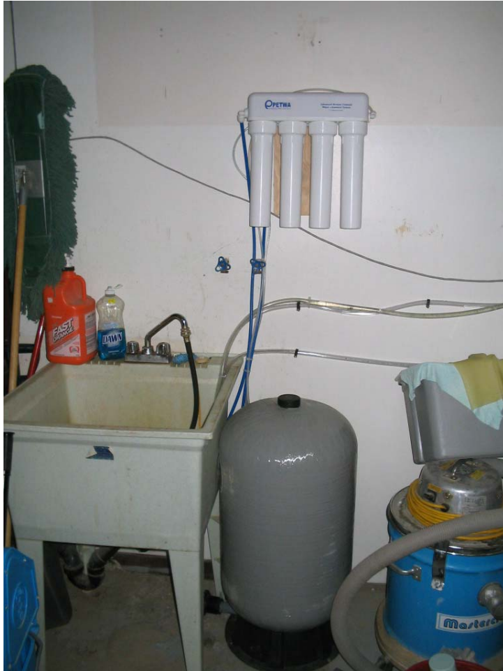
Photo 0004: 4840 Reverse osmosis system
