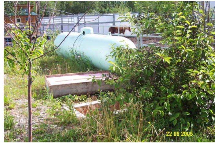
Photo 0310: 4976 Wellhead enclosure (centre), propane tank (behind), and horse corrals (back)
