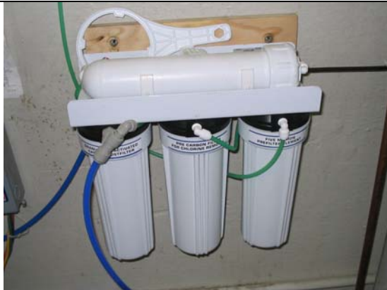
Photo 0011: 4981 Reverse osmosis system
