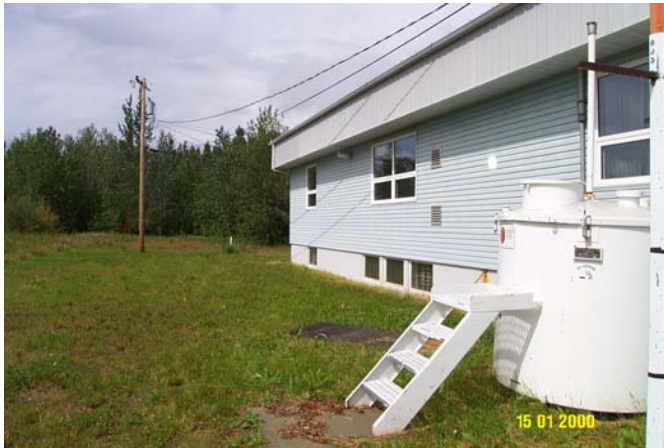
Photo 0272: 4981 Above ground fuel storage tank (right), EMR office (behind), and septic field (back left)
