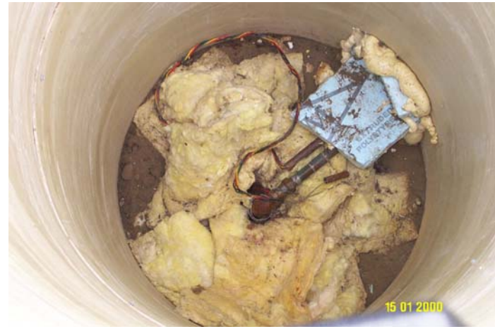
Photo 0269: 4981 Wellhead in pit
