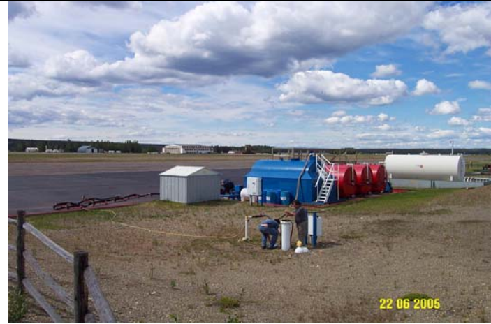
Photo 0318: 4993/4994 Pitless unit (front centre), above ground fuel storage tank (back right), fire retardant tanks (back right centre), chemical storage (back centre), and airport tarmac (behind)
