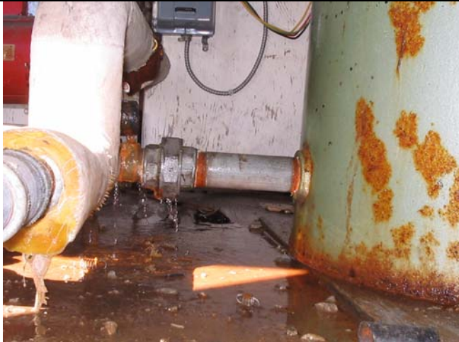
Photo 0055: 4873 Leak in piping from pressure tank
