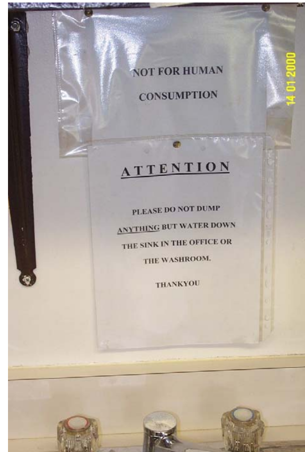
Photo 0228: 4793 Sign warning that water is not to be used as drinking water
