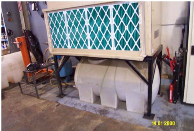
Photo 0231: 4793 Water storage tank
