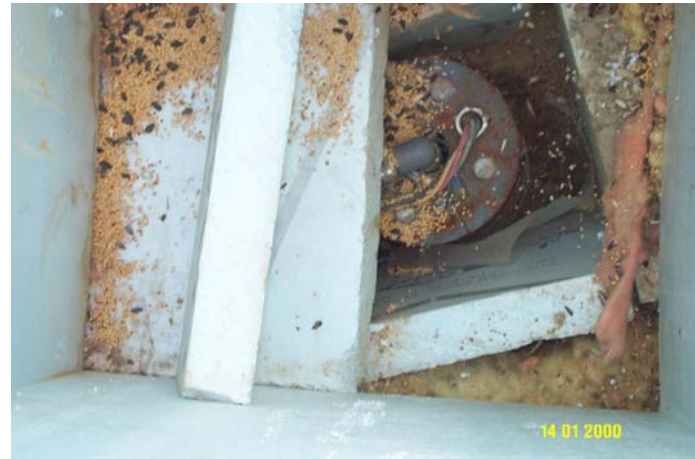
Photo 0237: 4799 Wellhead in pit
