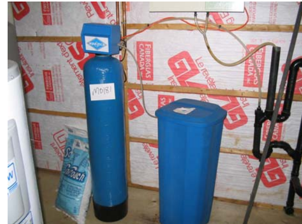
Photo 0025: M0181 Water softening system
