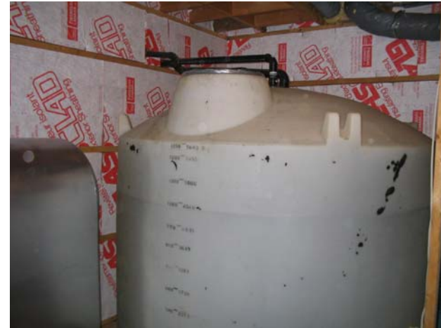
Photo 0022: M0181 5000 L water storage tank
