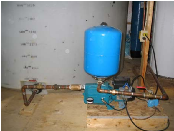
Photo 0023: M0181 Pressure tank
