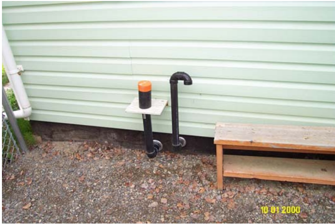
Photo 0215: M0181 delivery water fill
