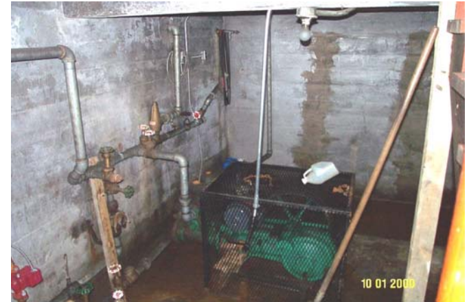
Photo 0221: 4782 Basement of Water Reservoir building. Water pump (centre), cistern behind left wall, note flooding on the floor.
