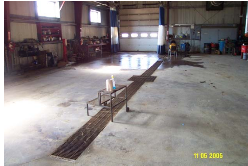
Photo 0134: Floor Drain System
