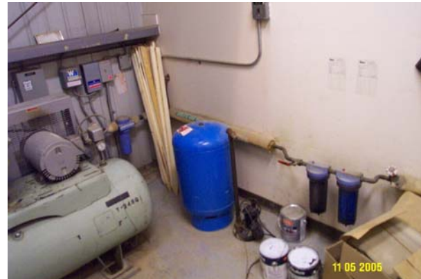
Photo 0136: Pressure Tank and Three In-Line Filters
