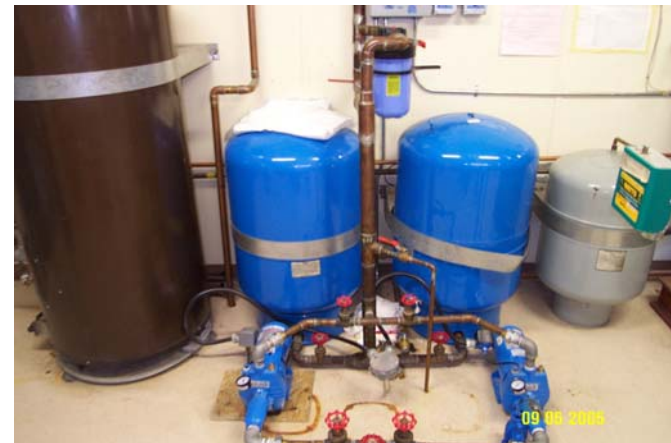
Photo 0086: 1322 Pressure Tanks and Filter
