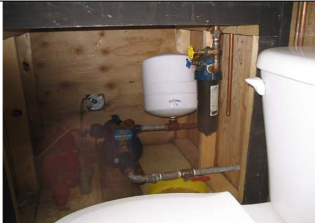
Photo 190: 5636 Jet pump and pressure tank.
