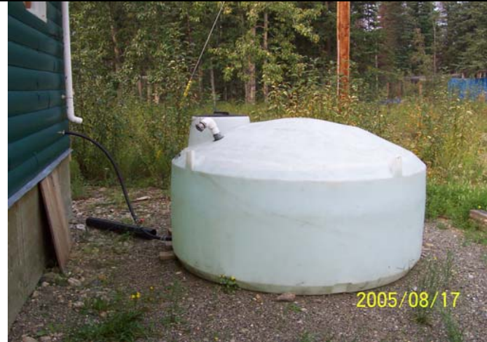
Photo 029: 5636 Seasonal water holding tank.
